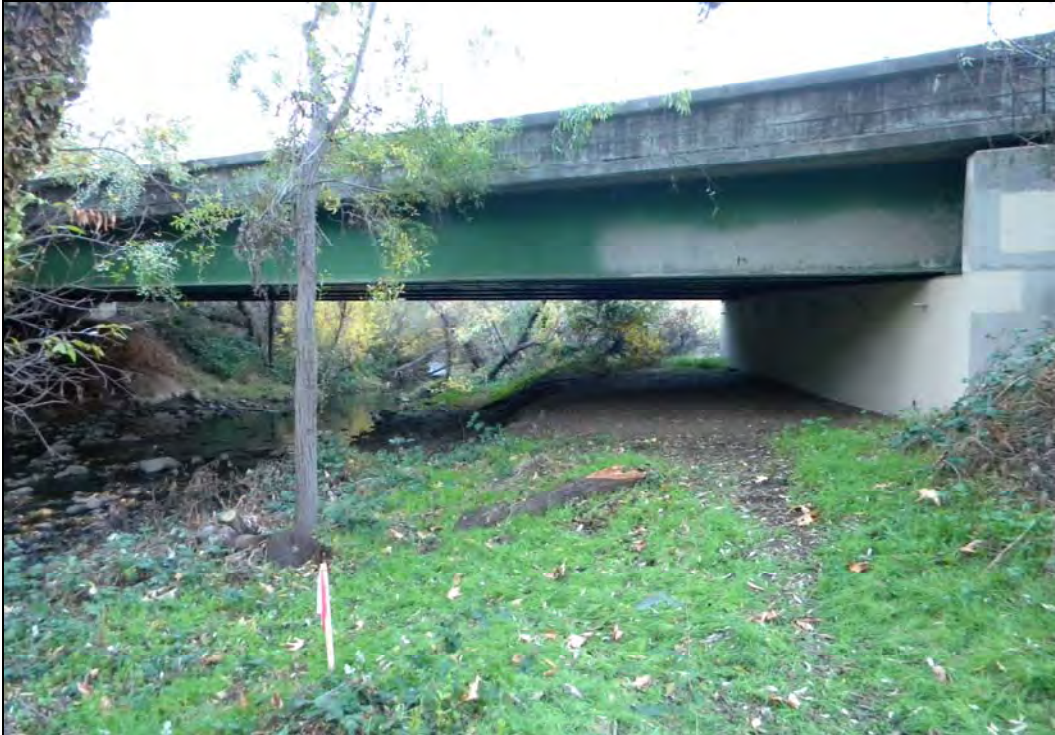
Figure 8: View southwest of Bridge 37C0160 with left (north) bank abutment to the right
