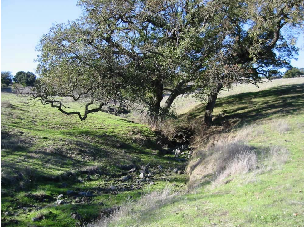
Stream Channel Erosion 2
