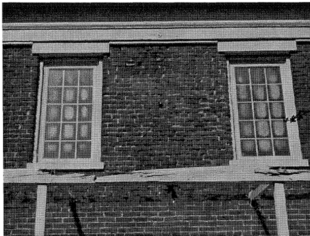
Deteriorated Brick at East Facade
